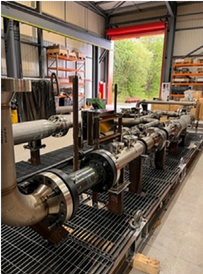
Flare gas recovery unit
